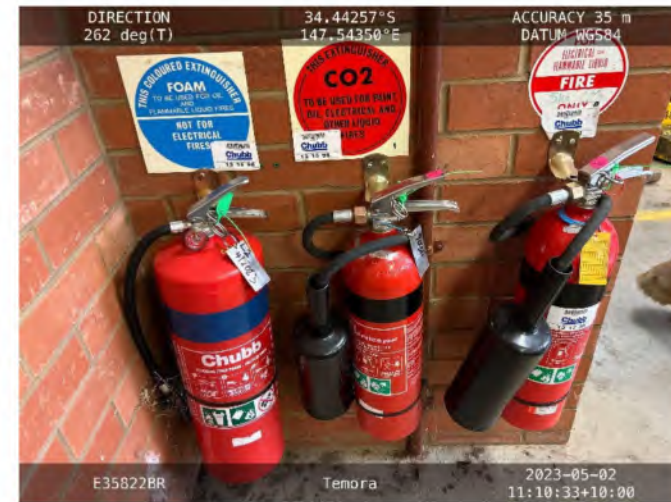
Photograph 6: Fire extinguishers in Maintenance building
