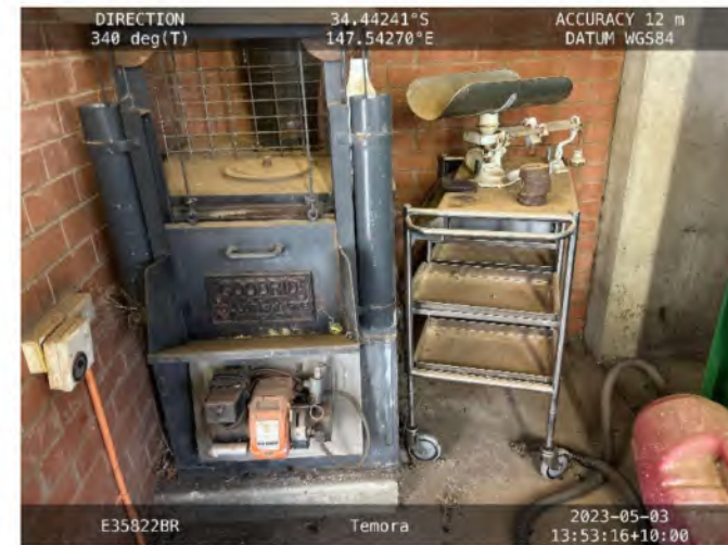
Photograph 8: Incinerator in Boiler room
