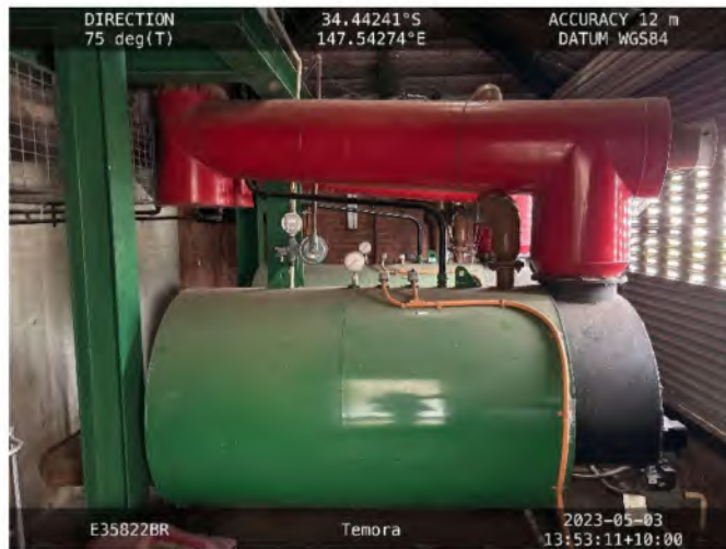
Photograph 7: Boilers in Boiler room
