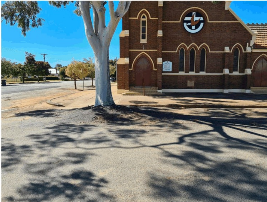
Image 1: Risen and Damaged pavement due to Gum tree roots.
