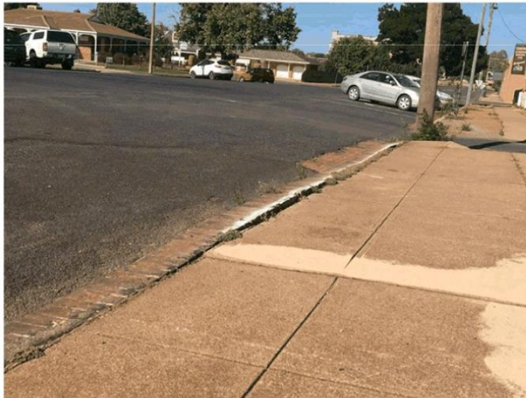
Photo 6 – Kerb and footpath defect
