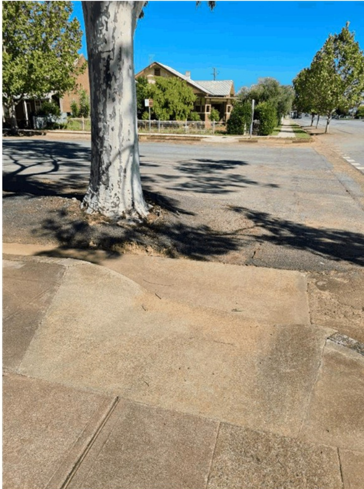
Image 3: Pedestrian access ramp is not parallel to opposite ramp.
