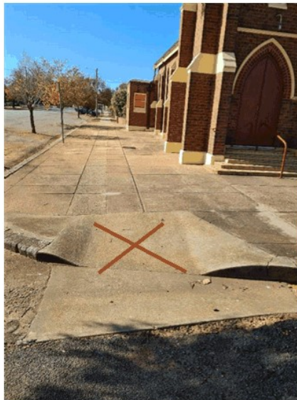
Image B: Remove existing kerb ramp on Eastern Side, reinstate kerb and gutter plus footpath behind
