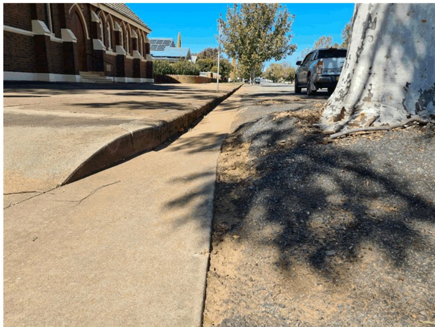
Image 2: Damaged pavement and gutter due to Gum tree.
